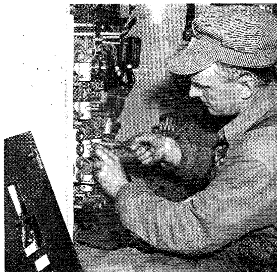
... and the automatic panel which operates the heating and cooling devices.
