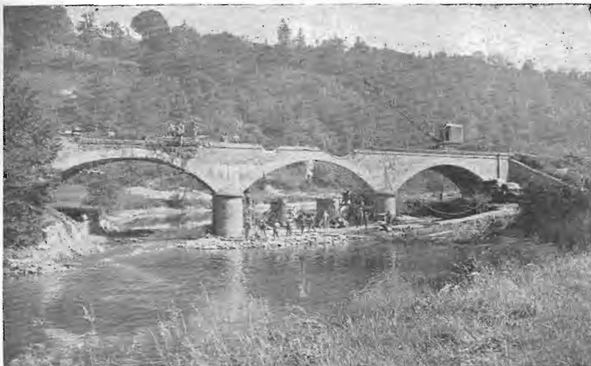
This is a fair example of what G.I. railroaders have been, and still are, up against in Europe. The men are shown at work repairing damage to a bridge just outside the French town of St. Lo. The middle section of the bridge has been almost completely torn apart.
